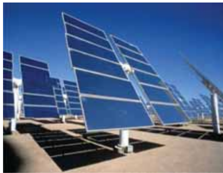
Figure 3: Photovoltaic power plant. Source: www.Nazeleno.cz .
