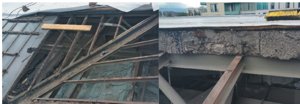
Figure 6: Degraded state of sheet metal and insulation under glass.
