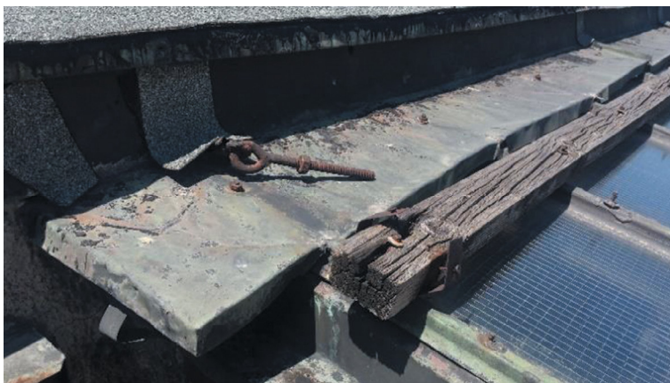
Figure 7: Remaining anchored parts.
