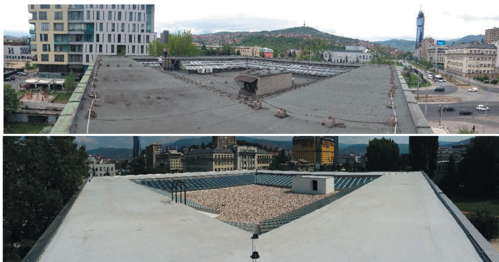
Figure 9: Condition of the roof (before and after).
