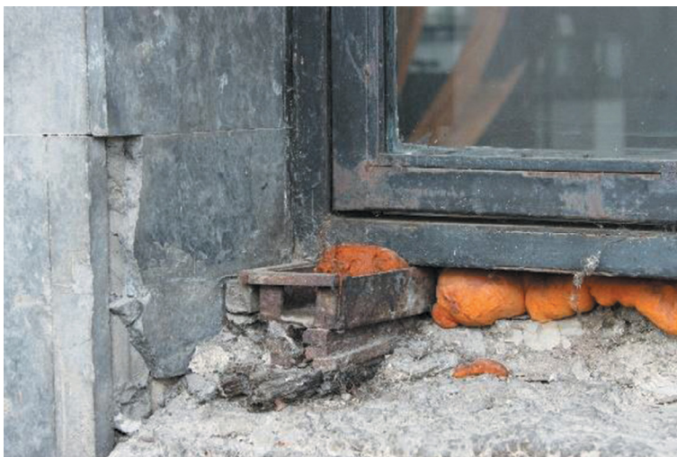
Figure 2: Ground floor openings that show improvised repairs.
